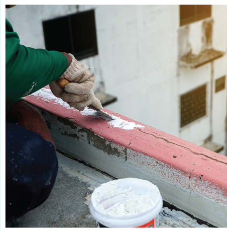
FOUNDATION CRACK REPAIR
